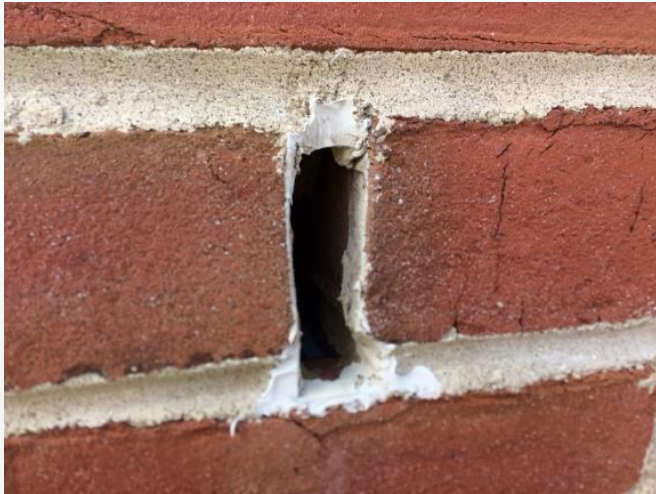
Evidence of Sealed Weep , Why?
