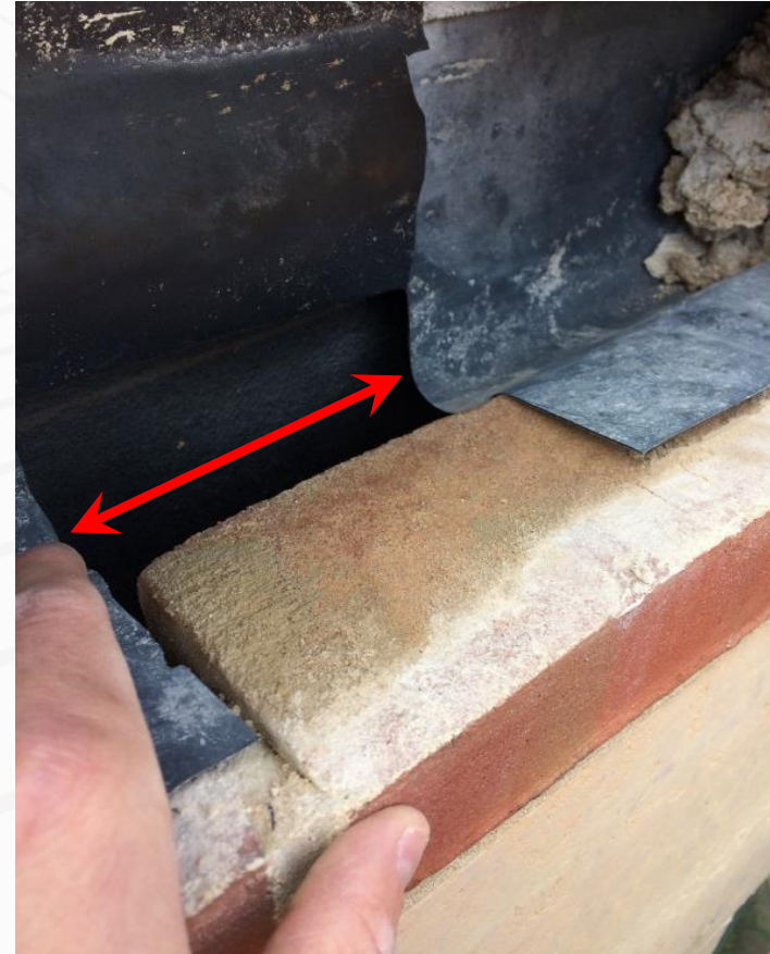
Incomplete Through Wall Flashing
