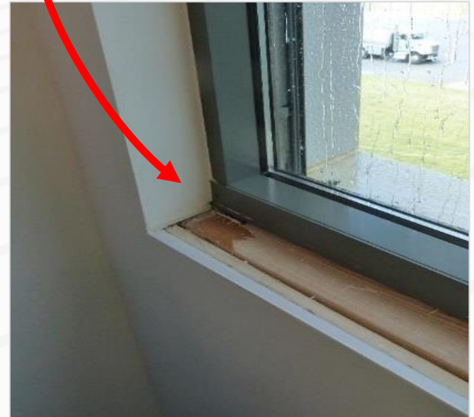
Water Testing Revealed Immediate Water Infiltration
