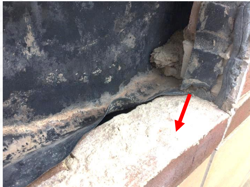
Breach in Drainage Plane
