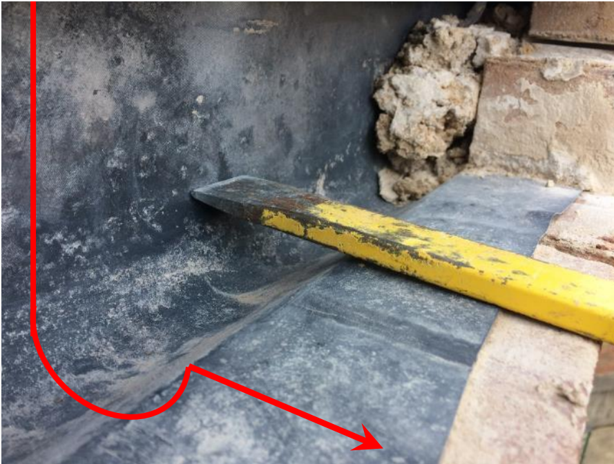
Improper Through Wall Flashing Installation – Water Cannot Escape From Drainage Plane
