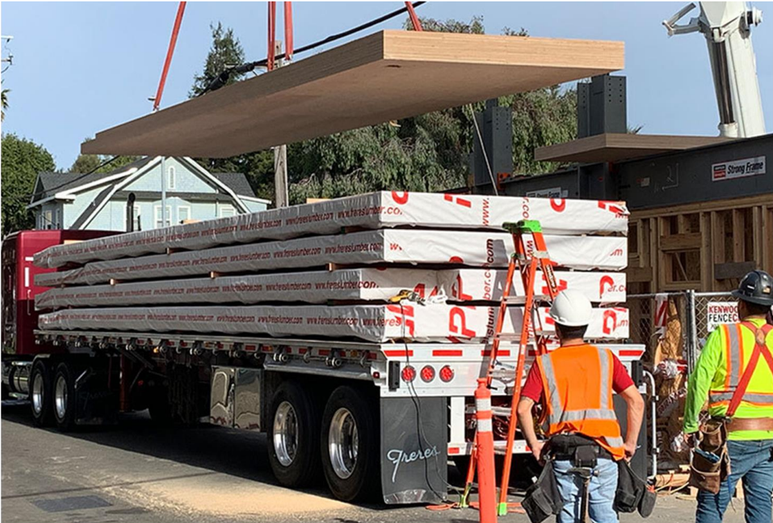
Mass timber is trucked to site as required typically 1-3 trucks a day to keep a steady flow of materials
