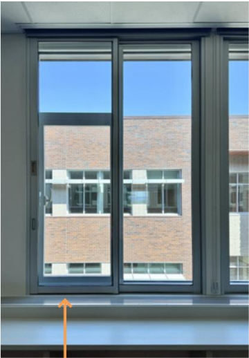
When both windows are closed, exterior sound is blocked
